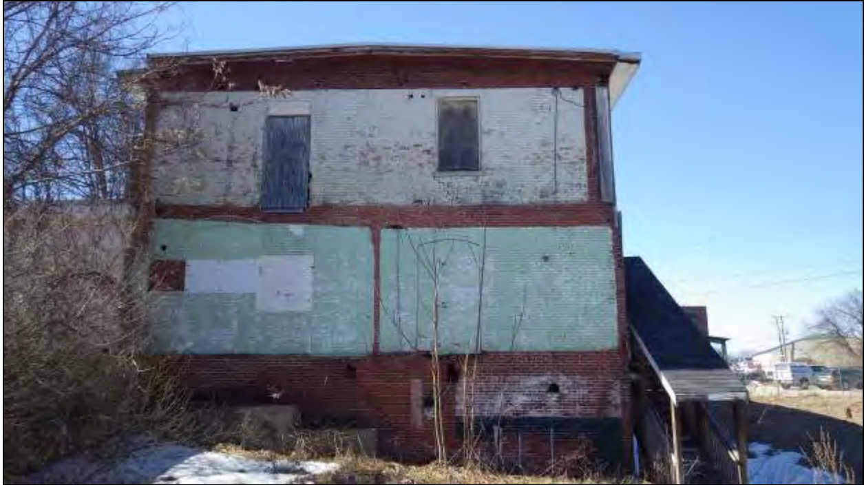
Figure 89 - South wall of an old building, facing northwest toward Crown Street. Ghost marks of the demolished building are visible on the south façade of the Armstrong building.
