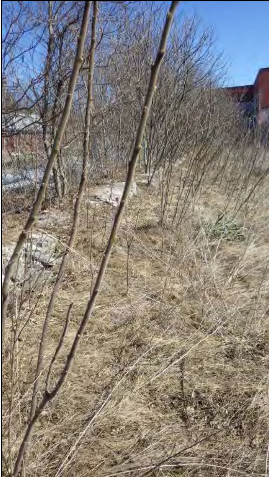
Figure 84 - Stone foundation paralleling tracks that formed the north wall of a demolished structure, facing southeast.
