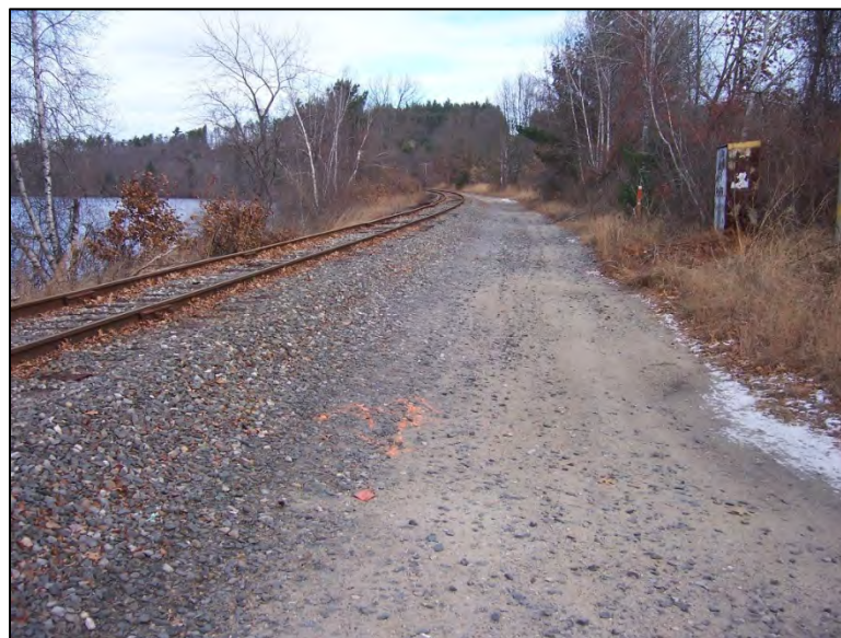
View north of the existing rail line and the Merrimack River near Depot Road in Hooksett
