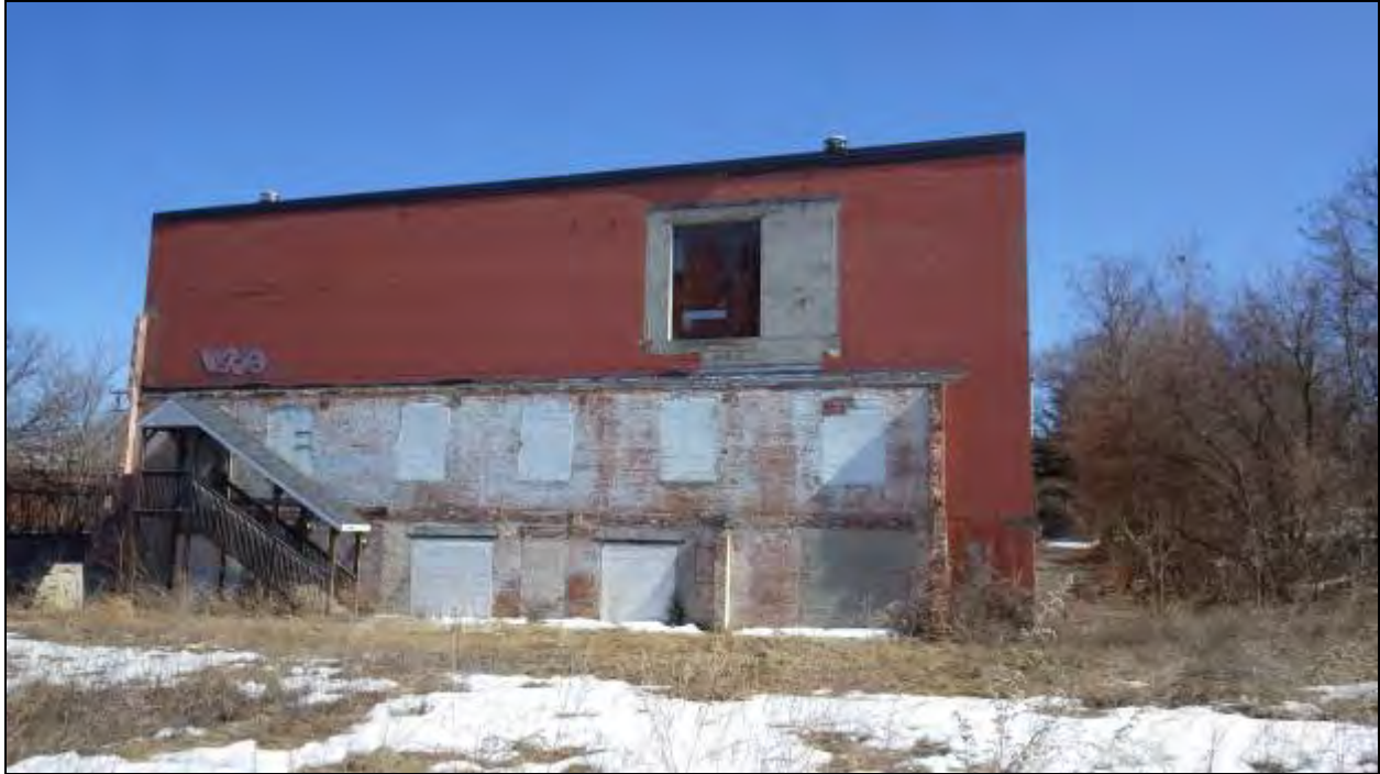
Figure 92 - North wall of an old manufacturing/warehouse building. A modern cinderblock story was added on top of the original brick two-level warehouse.
