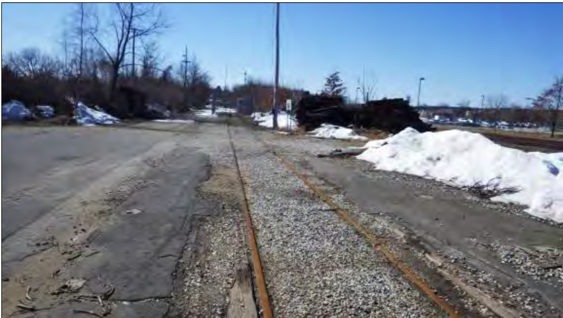
Photo 10. Proposed Granite Street layover location; view south along the right-of-way from the north end of the limits of disturbance
