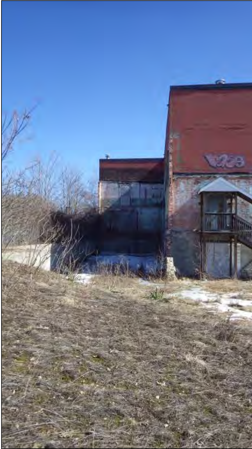
Figure 91 - North wall of an old factory building, now destroyed and acting as an alcove, facing southeast. In the left of frame is a berm of soil and debris along the western edge of the large demolished building.
