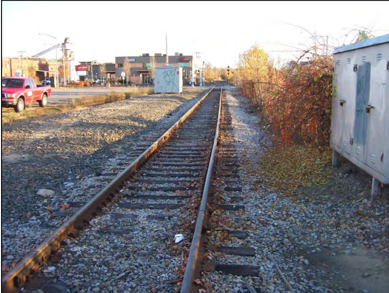
View south along existing rail line at Granite Street Station Site in Manchester
