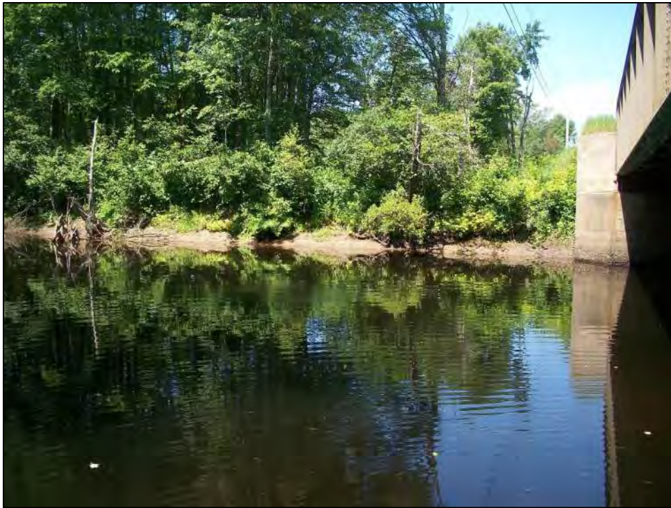
Photo 3. View northwest of the Blackwater River and bank in the southwest bridge quadrant (Impact Areas H, I, and J). Photo taken on 7/19/2019.
