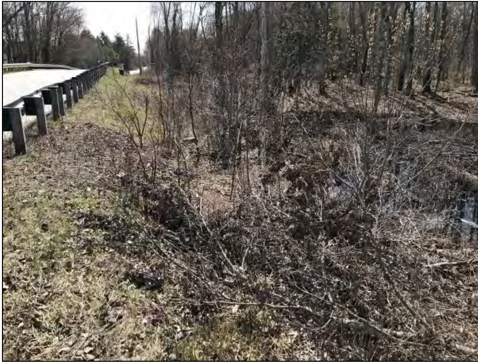
Photo 7. View southeast toward Impact Area C (Wetland 2), located in the southwest bridge quadrant. Photo taken on 4/21/2023.
