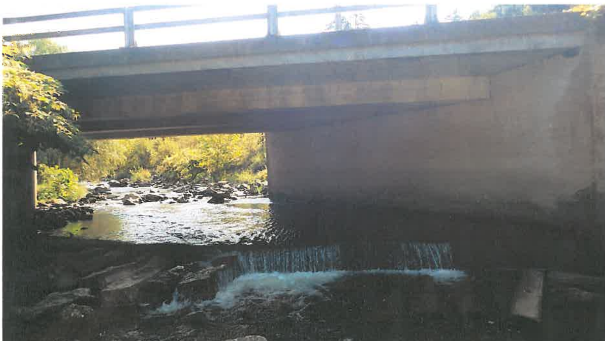
Figure 4. Impact Areas C, E and H: View of Warren Brook looking upstream (east) through the crossing, including the existing granite slabs and perch at the outlet and the existing concrete pad, from downstream (west) of Bridge 073/163. Proposed channel impacts due to removal of granite slabs, concrete pad and abutments, work access and installation of BMPs. (Meli Dube, September 2017)
