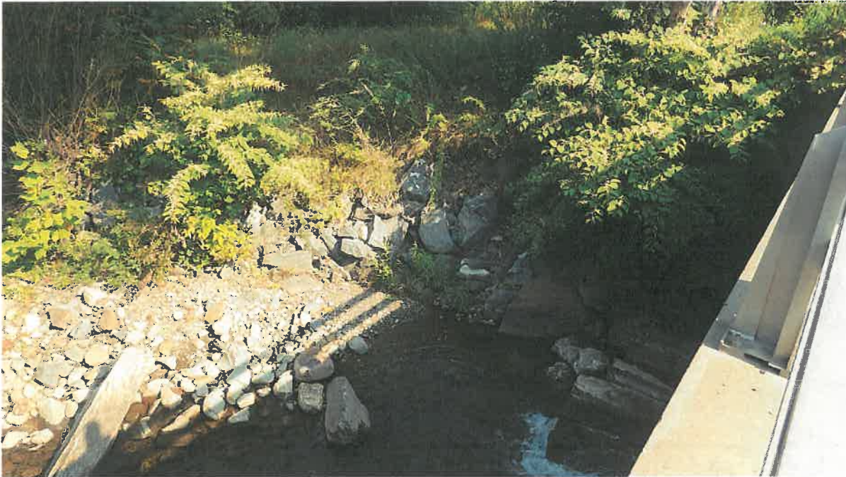
Figure 7. Impact Areas C, B and A: View of downstream channel and bank in the northwestern quadrant of the crossing from Bridge 073/163. Proposed bank impacts due to removal of wingwall and grading to match downstream slope, proposed channel impacts due to removal of granite slabs, work access and installation of BMPs. (Meli Dube, September 2017)
