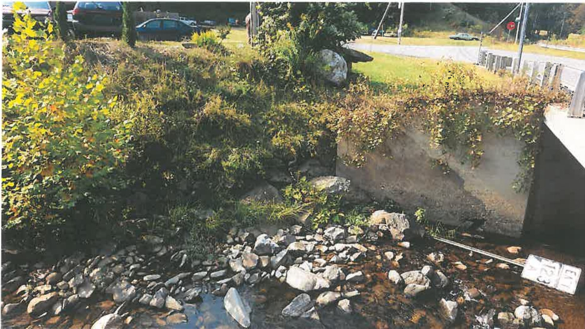
Figure 5. Impact Areas H, J and I: View of the upstream channel and bank in the southeastern quadrant of the crossing from the upstream bank in the northeastern quadrant. Proposed bank impacts due to removal of wingwall and grading to match upstream slope, channel impacts due to work access and installation of BMPs. (Meli Dube, September 2017)
