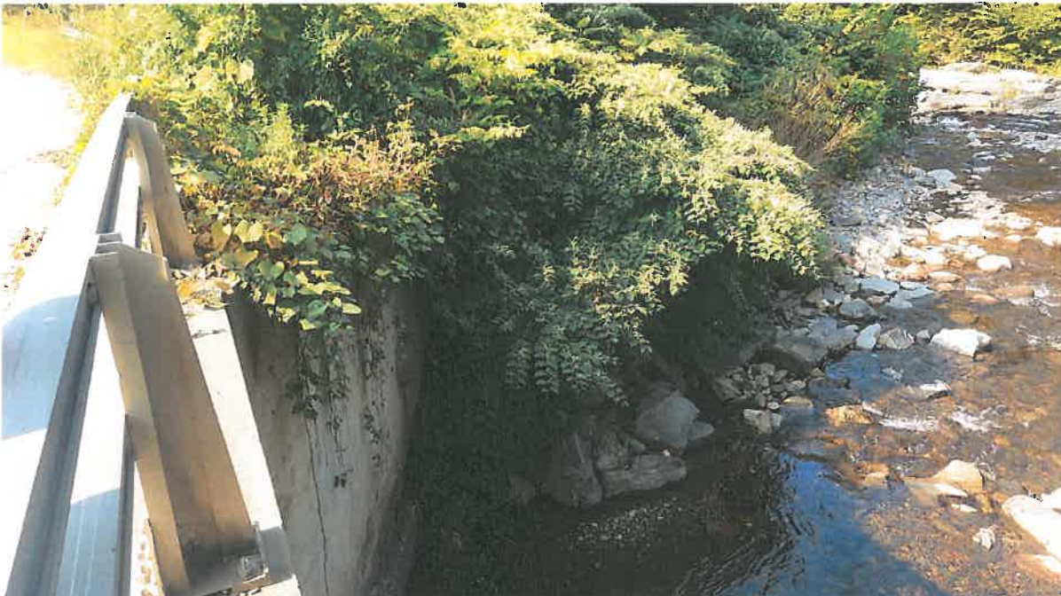
Figure 8. Impact Areas C and D: View of downstream channel and bank in the southwestern quadrant of the crossing from Bridge 073/163. Proposed bank impacts due to removal of wingwall and grading to match downstream slope, proposed channel impacts due to work access and installation of BMPs. (Meli Dube, September 2017)
