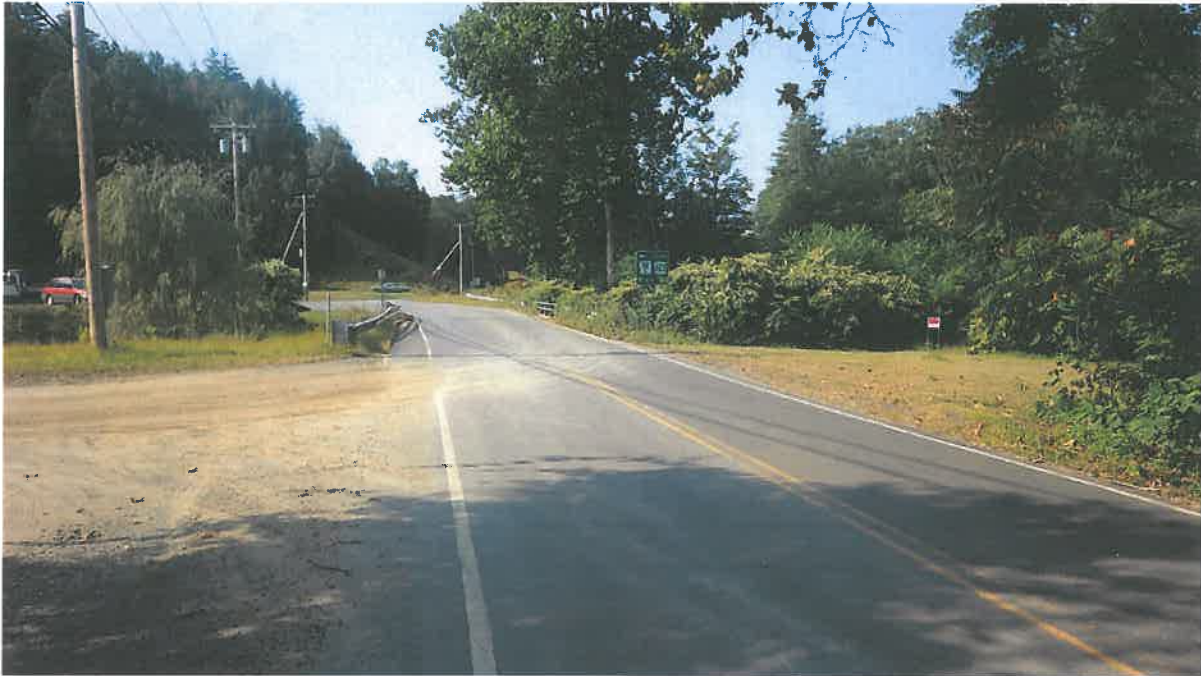
Figure 1. View of project area looking south towards NH Route 123/NH Route 12 from north of Bridge 073/163 on NH Route 123A. (Meli Dube, September 2017)
