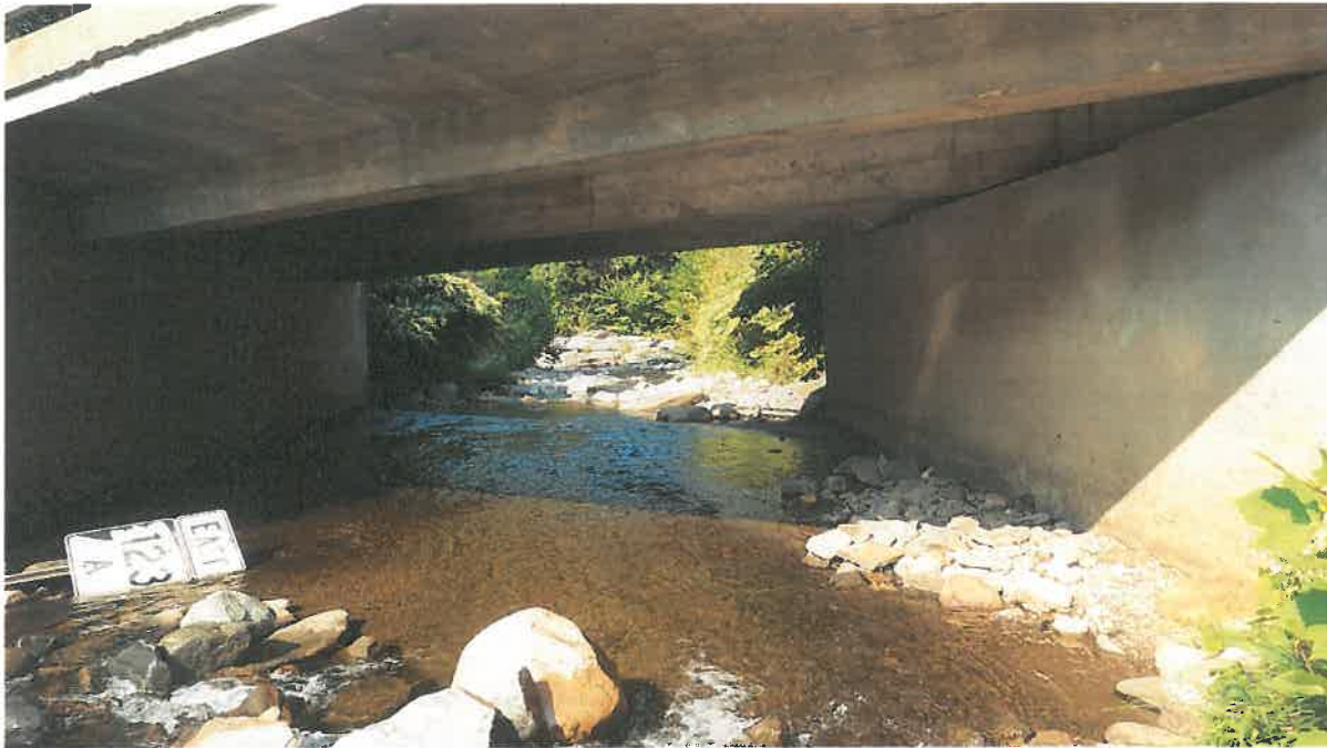
Figure 3. Impact Areas E and C: View of Warren Brook looking downstream (west) towards the confluence of the Cold River through the crossing, including the existing concrete pad, from upstream (east) of Bridge 073/163. Proposed channel impacts will be due to removal of the concrete pad and existing abutments, work access and installation of BMPs. (Meli Dube, September 2017)
