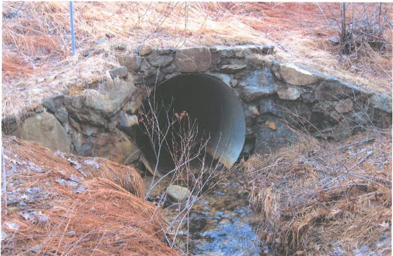
Figure 8. Impact Location F: Outlet side of 66" pipe, Wetland P8. Photo taken by the NHDOT Bureau of Environment on 4/13/18.
