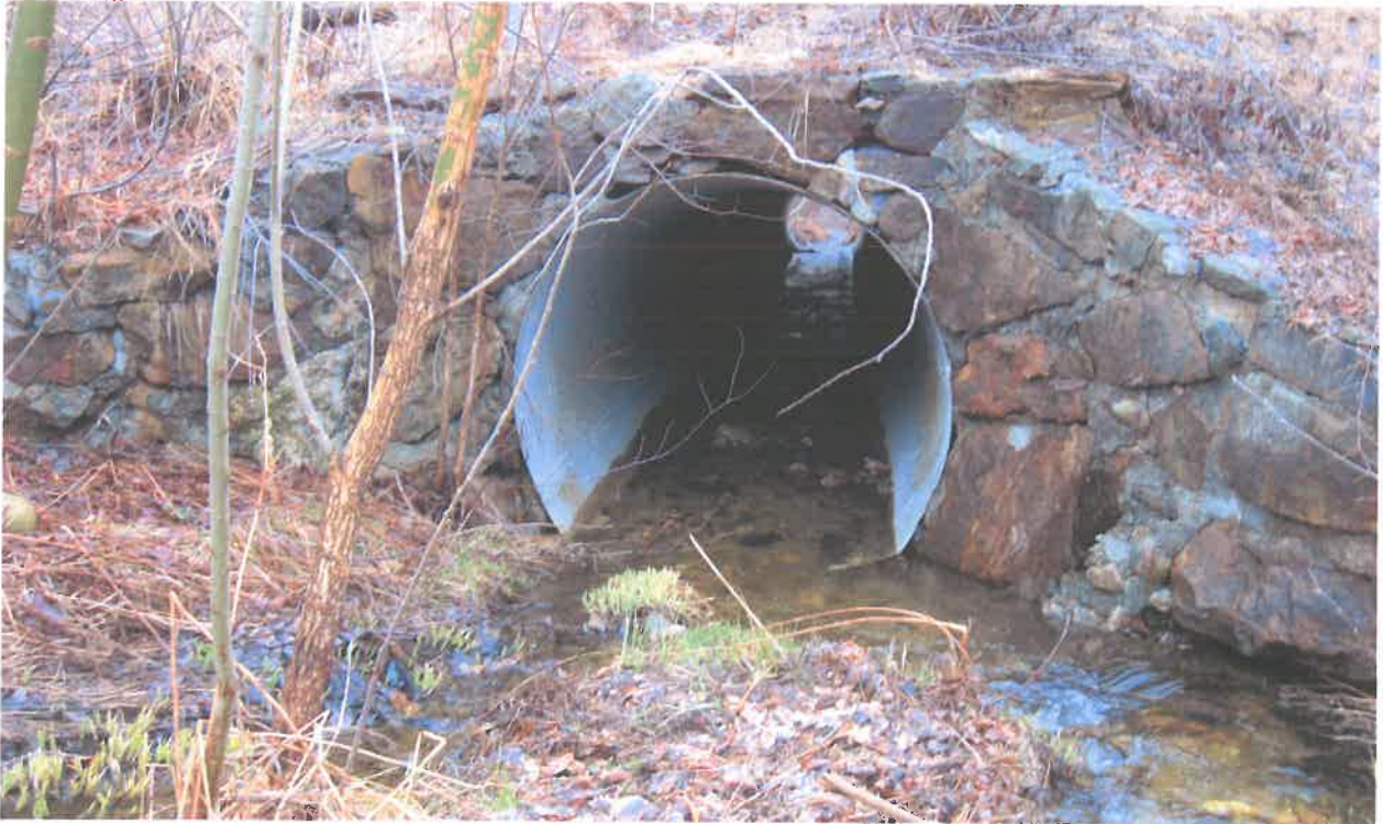
Figure 5. Impact Location D: 66" pipe inlet, Wetland P8. Photo taken by the NHDOT Bureau of Environment on 4/13/18.
