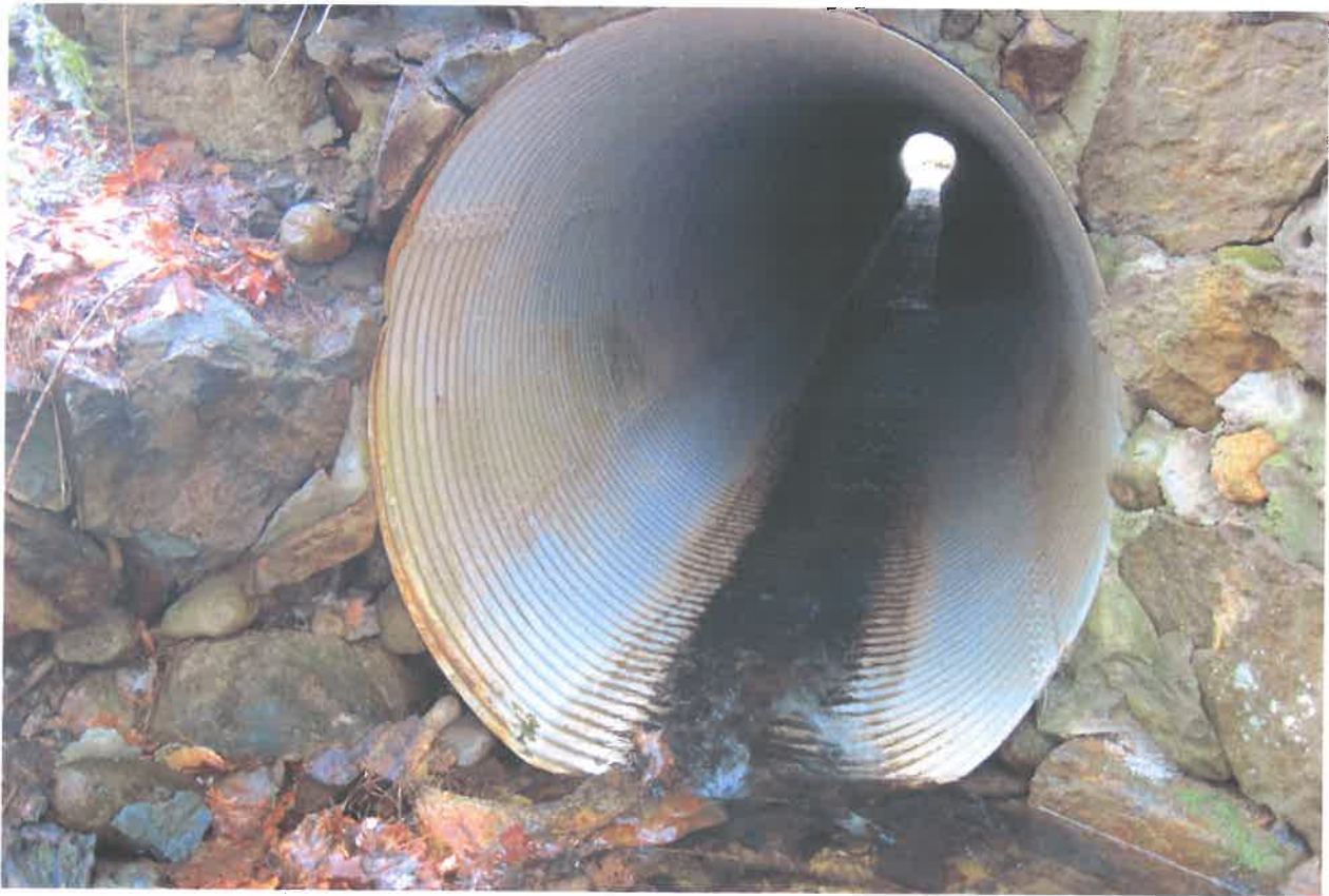
Figure 2. Impact Location B: inside of 60" pipe, inlet side, Wetland P1. Photo taken by the NHDOT Bureau Of Environment on 4/13/18.
