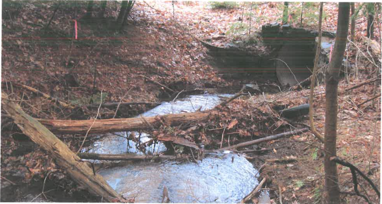
Figure 1. Impact Location A: Looking downstream toward 60" pipe inlet, Wetland P1. Photo taken by the NHDOT Bureau of Environment on 4/13/2018.
