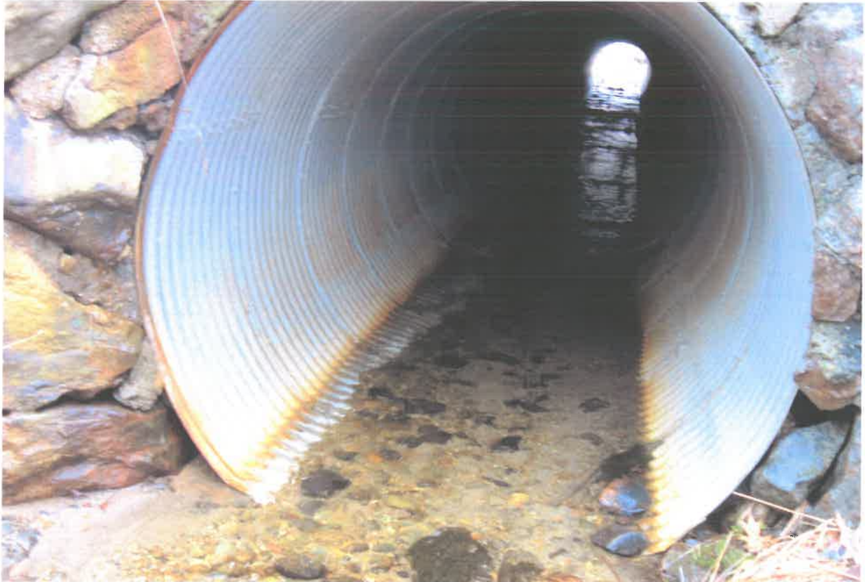
Figure 7. Impact Location E: Inside 66" pipe, looking from outlet side, Wetland P8. Photo taken by the NHDOT Bureau of Environment on 4/13/18.
