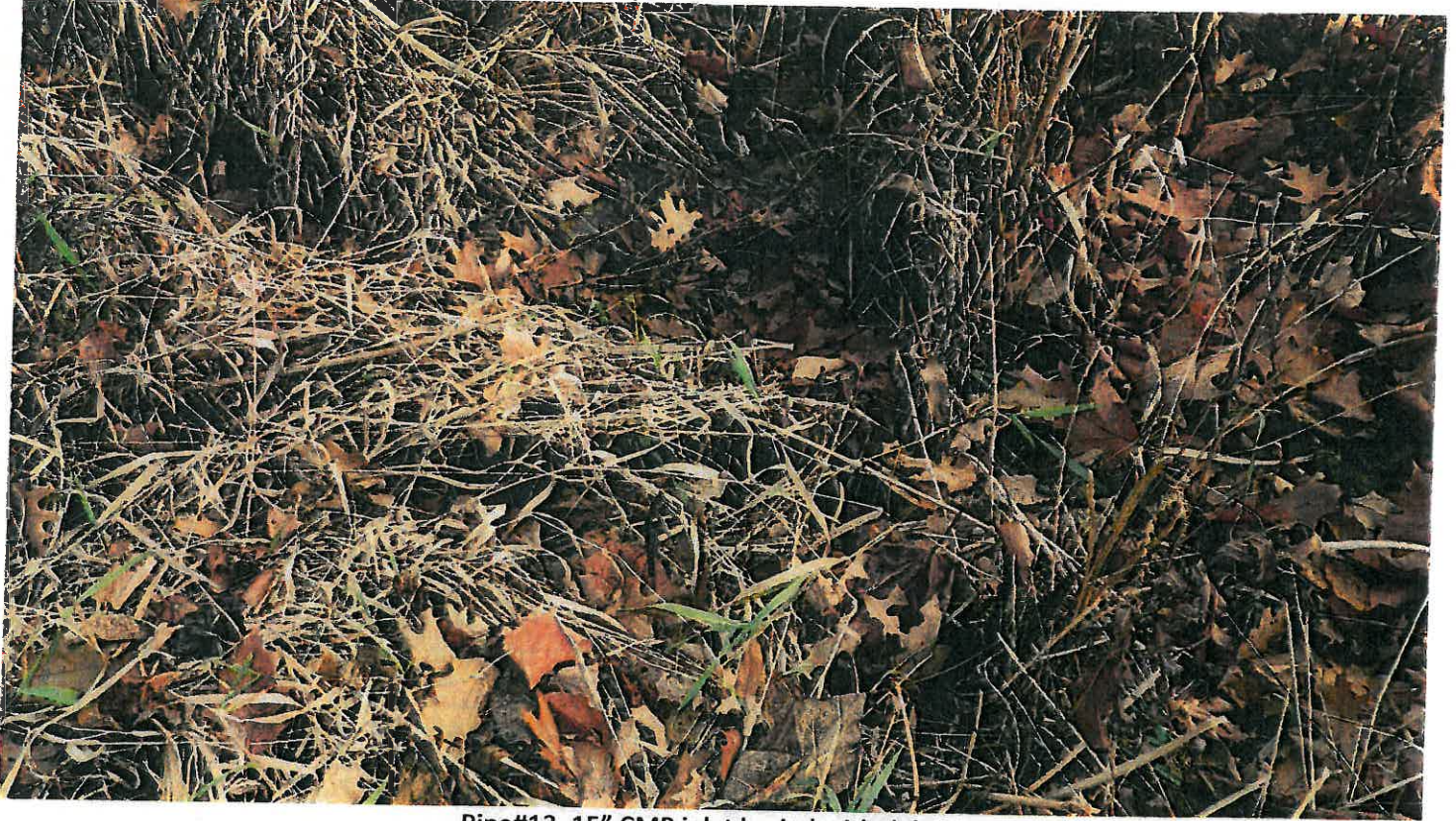
Pipe#13, 15" CMP inlet buried with debris.
