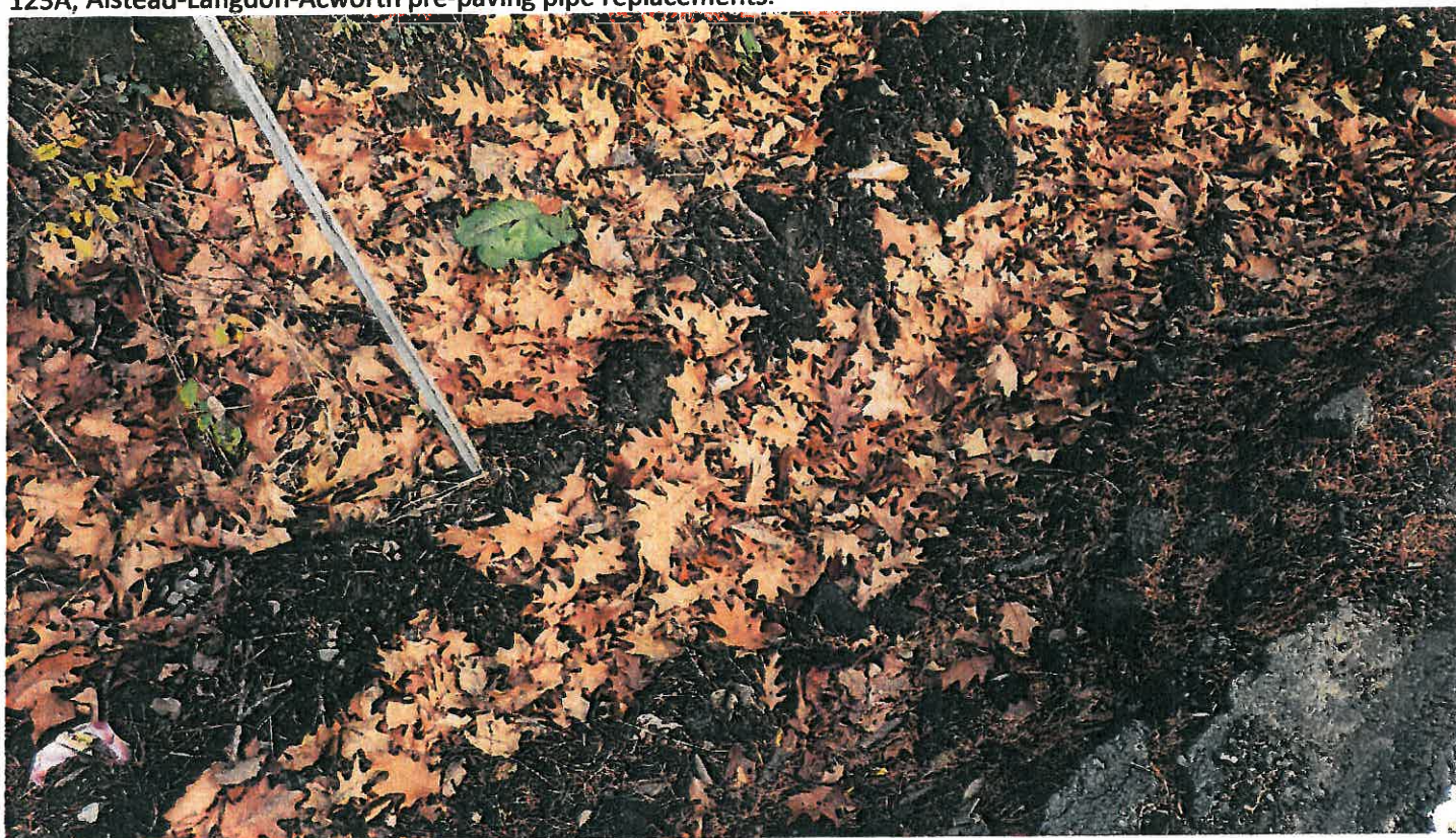
Pipe #14, 15" CMP inlet covered with debris.
