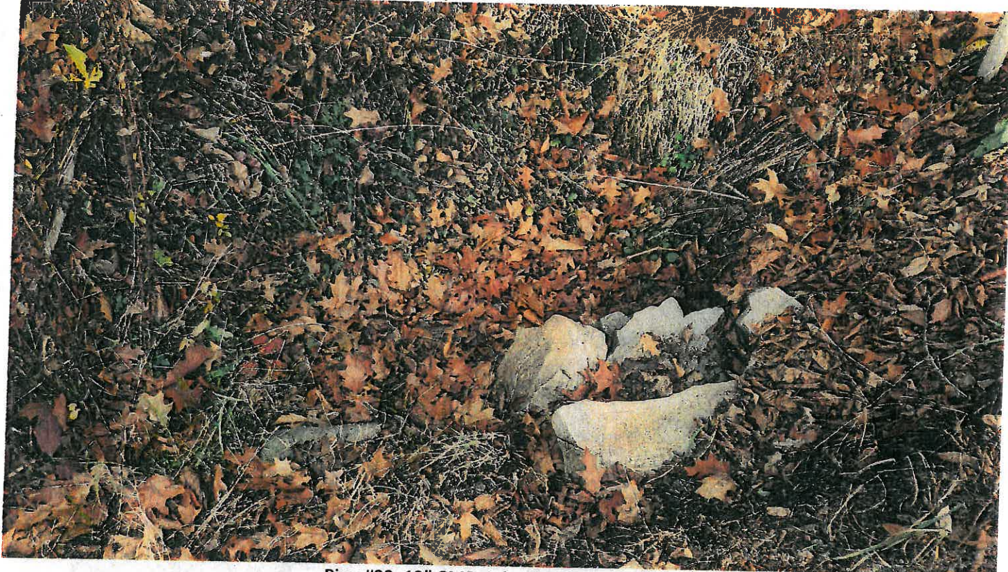
Pipe #22, 12" CMP, Inlet Header collapsed.
