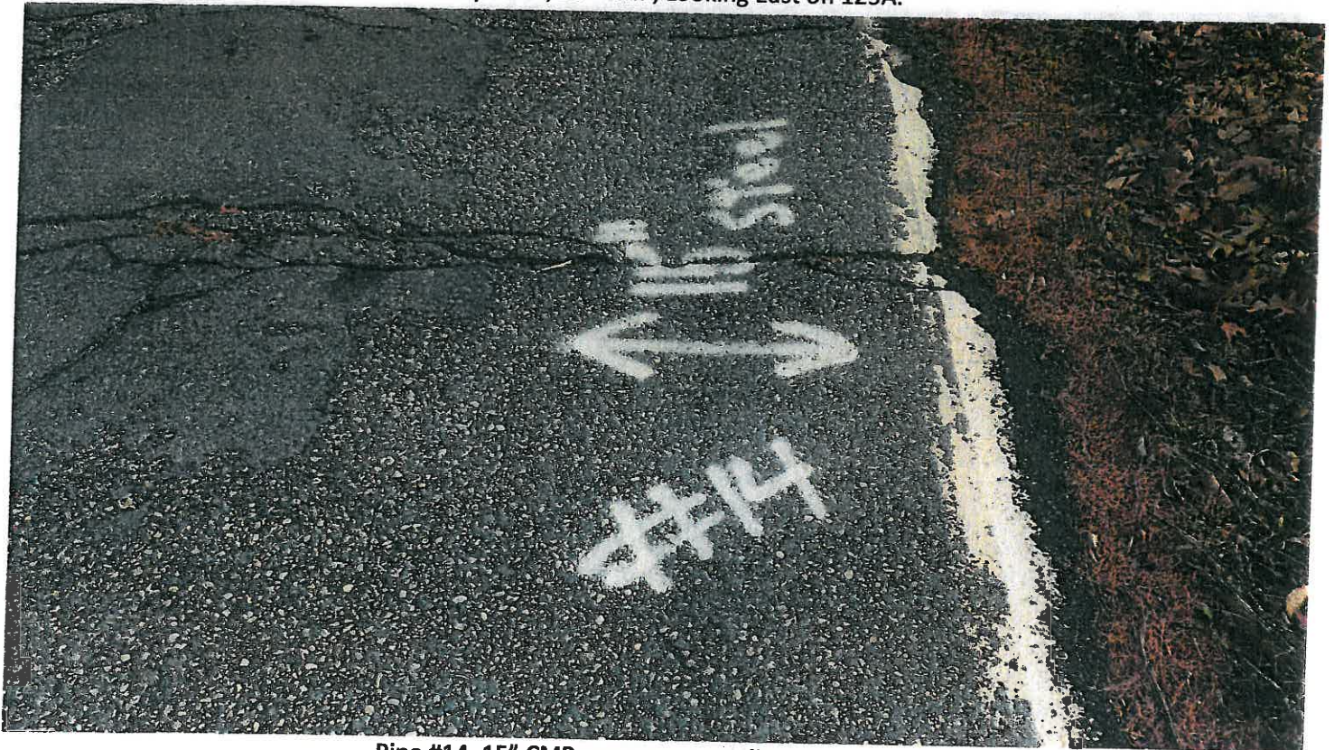
Pipe #14, 15" CMP, pavement condition at crossing.
