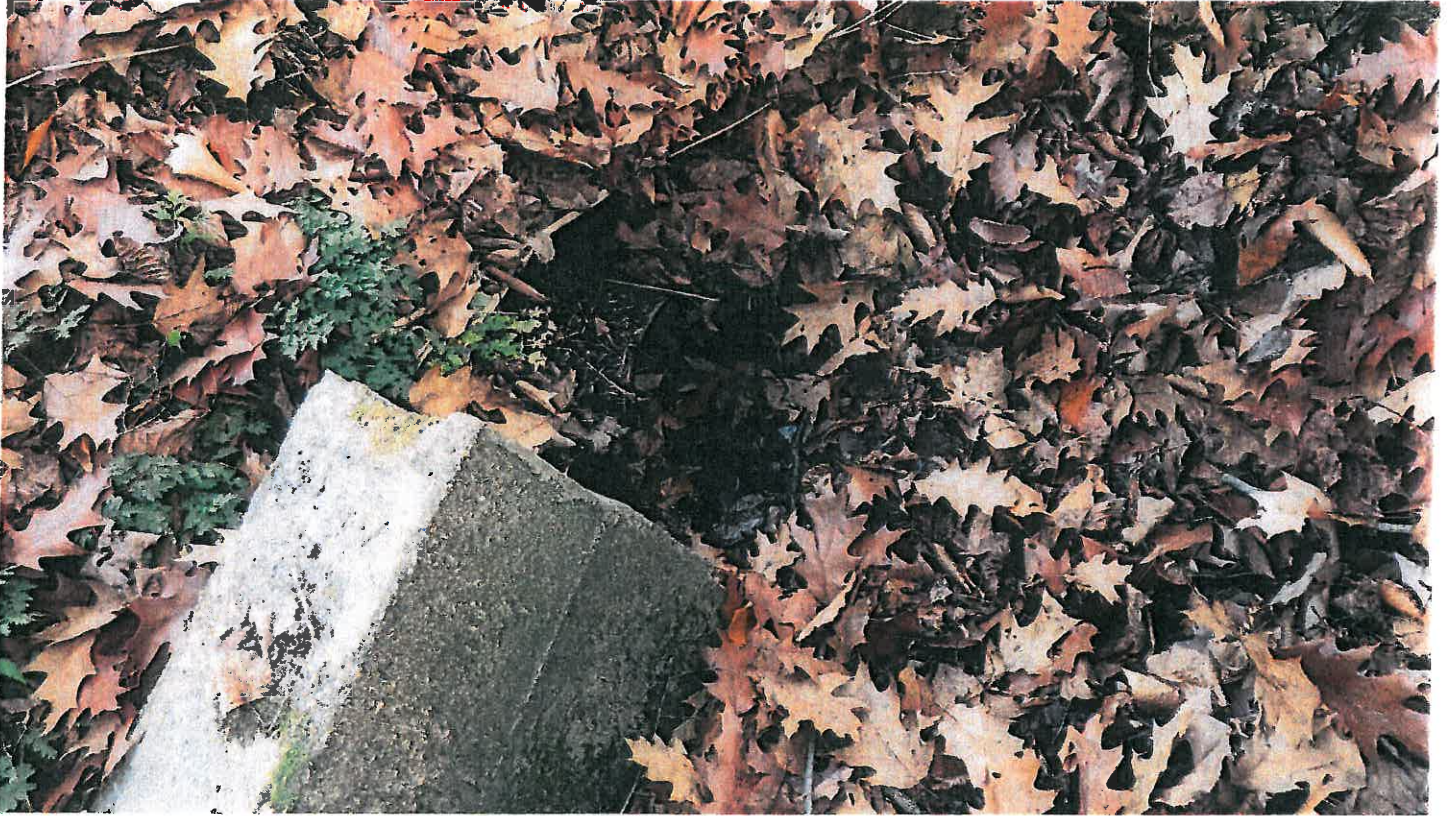
Pipe#7, 15" RCP, inlet.
