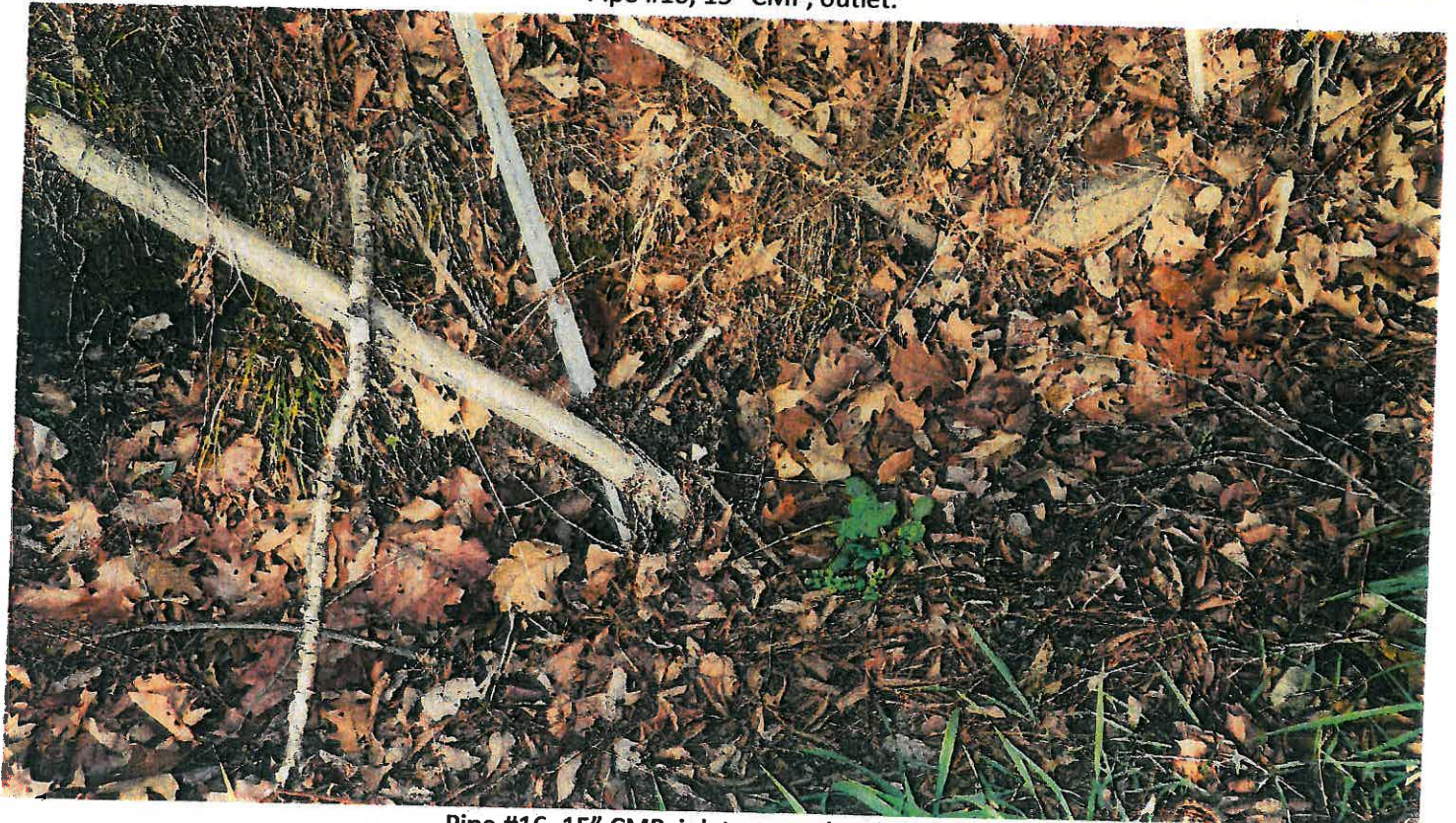
Pipe #16, 15" CMP, inlet covered with leaves.
