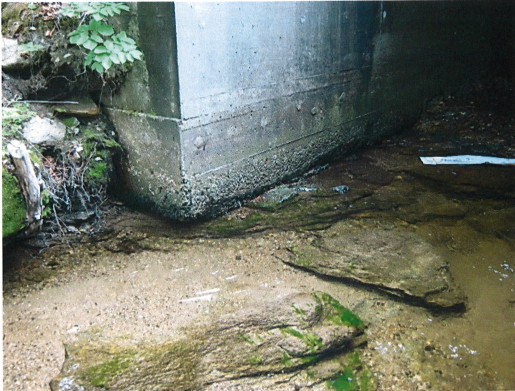
Figure 3: Voids between east abutment and ledge at north (6/2014).
