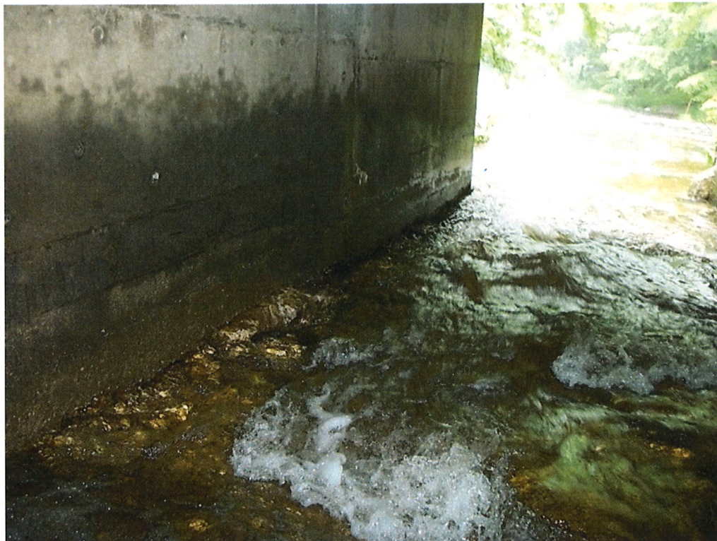
Figure 4: Scour at west abutment (6/2012).
