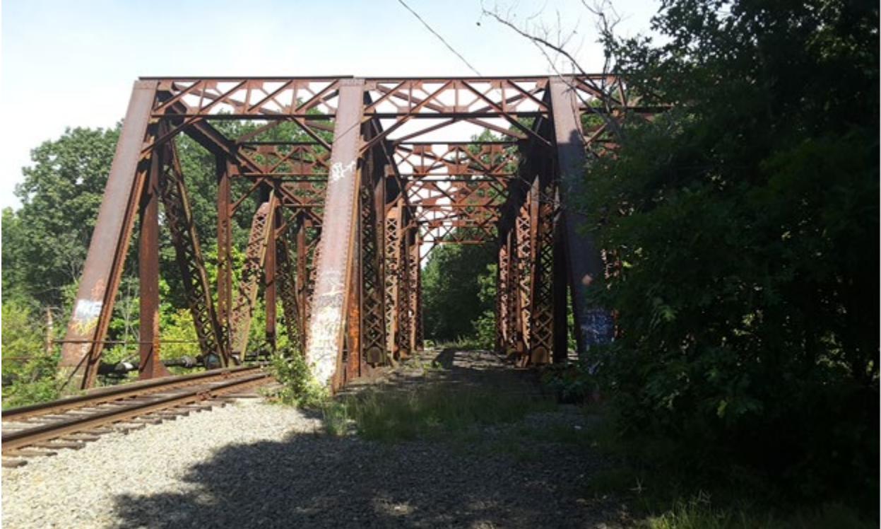
Photo 27. A view looking northwest showing a close-up perspective of the ca. 1900 bridge BR#71 #39.22 (CCP-016) where it crosses the Nashua River in Nashua.
