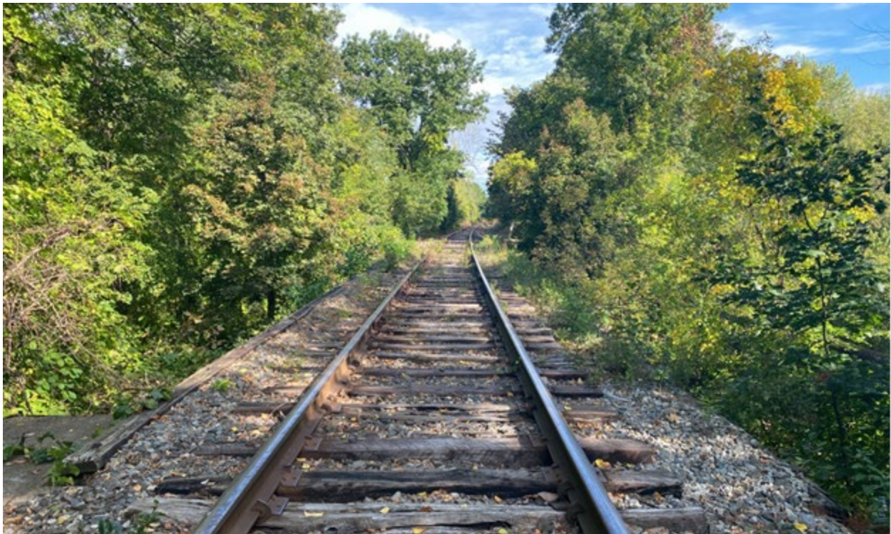
Photo 20. A view looking north across ca. 1844 bridge #78 #44.92 (CCP-012) where it crosses the Naticook Brook in Merrimack.
