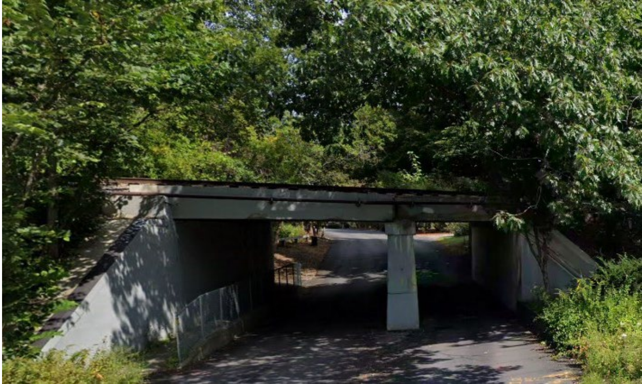
Photo 25. A view looking east showing a close-up perspective of the bridge tunnel, BR#72 #39.39 (CCP-015).
