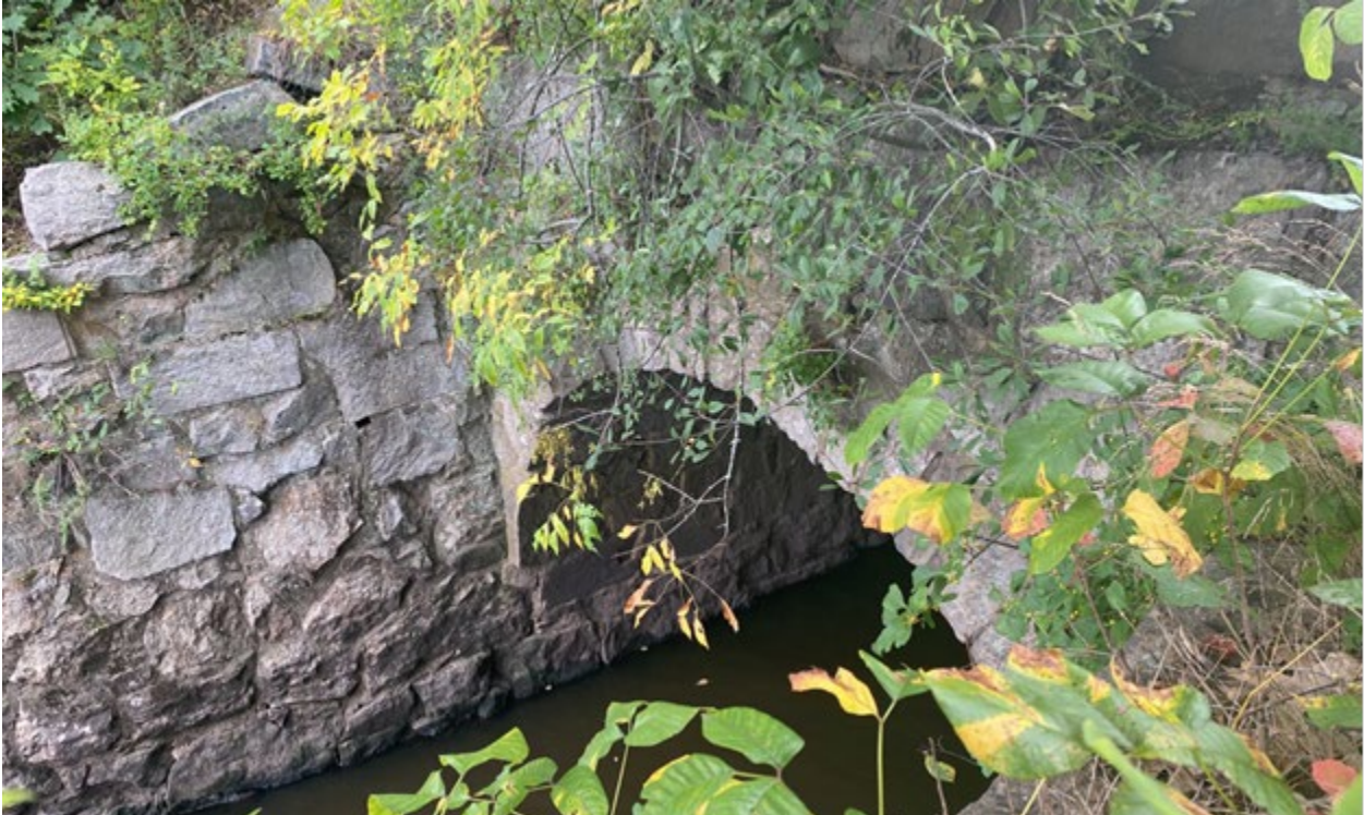
Photo 39. A view looking southwest showing the east side of the ca. 1848-1850 stone arched railroad bridge BR#70 #37.87 (CCP-025) where it crosses Salmon Brook in Nashua.
