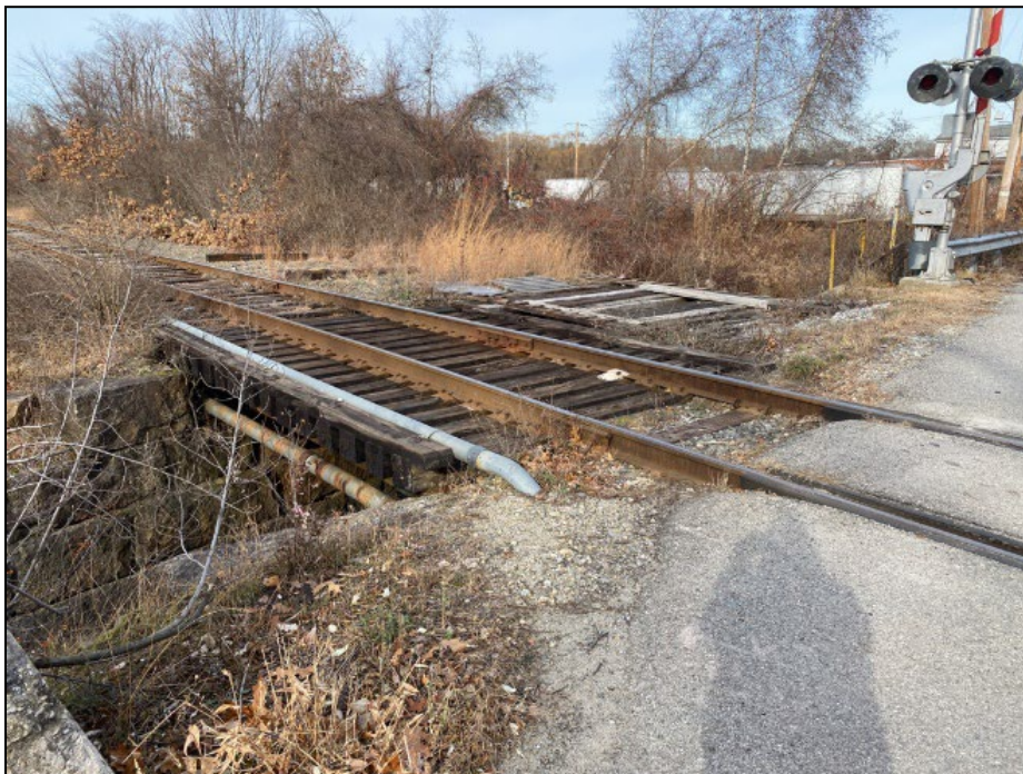
Photo 6. View of top of Wotton Rd - Deep Brook Railroad Bridge (CLM.920), looking north.
