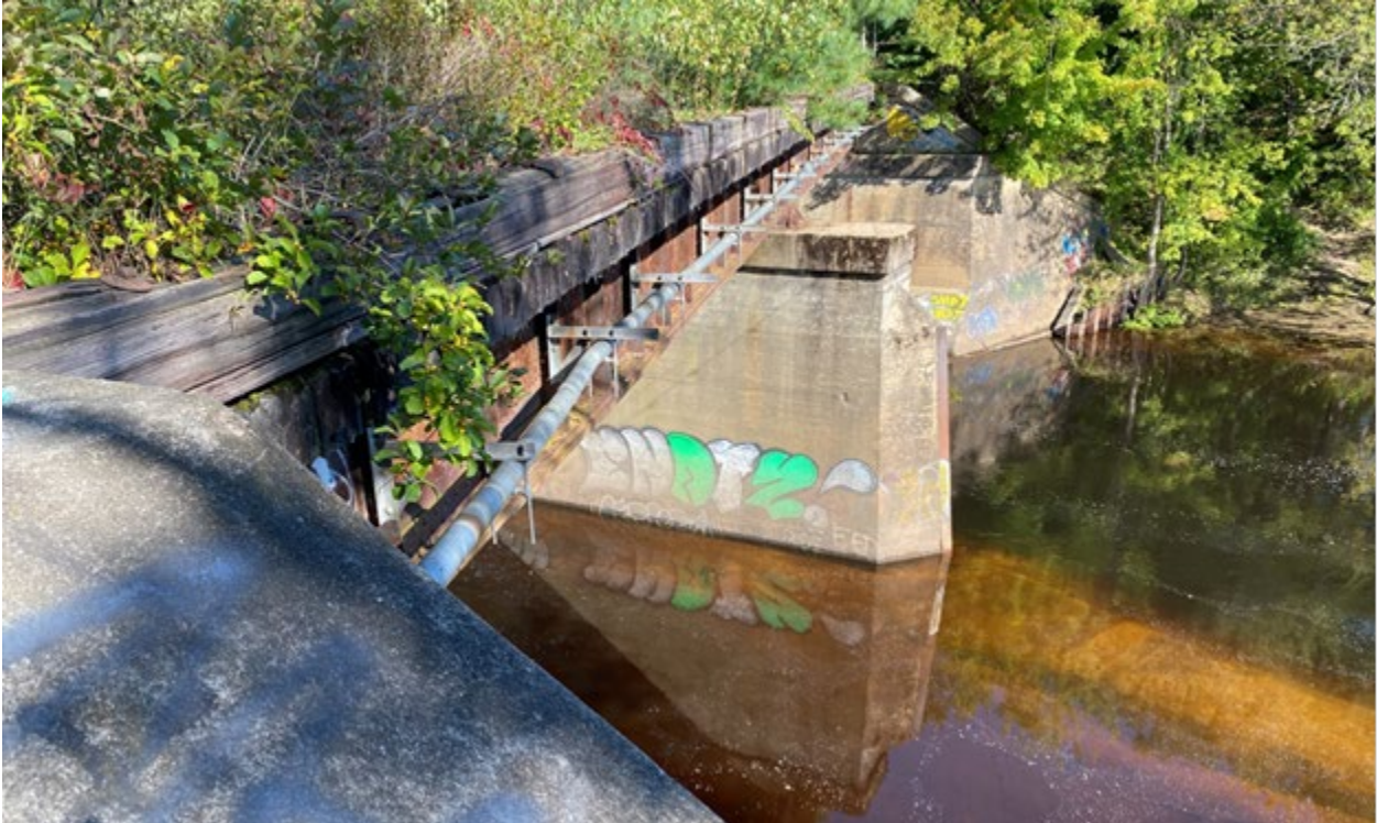
Photo 17. View looking northwest showing the east side of pre-1947 bridge BR#79 #46.22 (CCP-011) where it crosses the Souhegan River in Merrimack.
