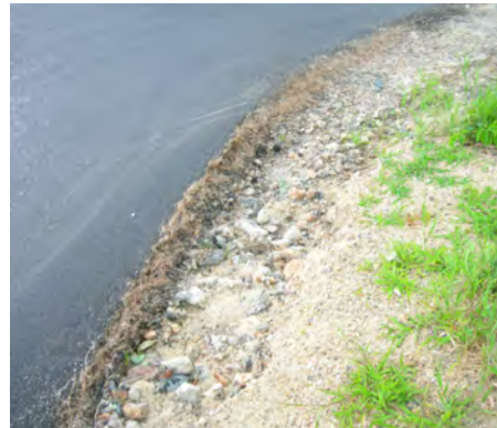
Photo 5.3.4 Pavement Edge Drop-off
