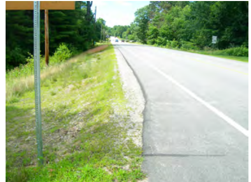
Photo 5.4.5 Pavement Edge Drop-off
