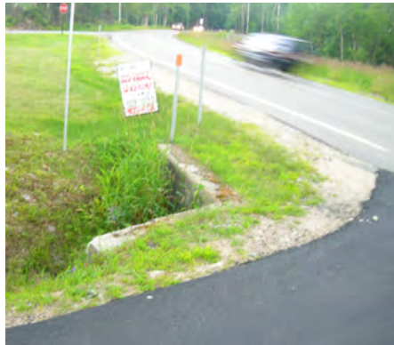
Photo 5.3.3 Hazard in Clear Zone
