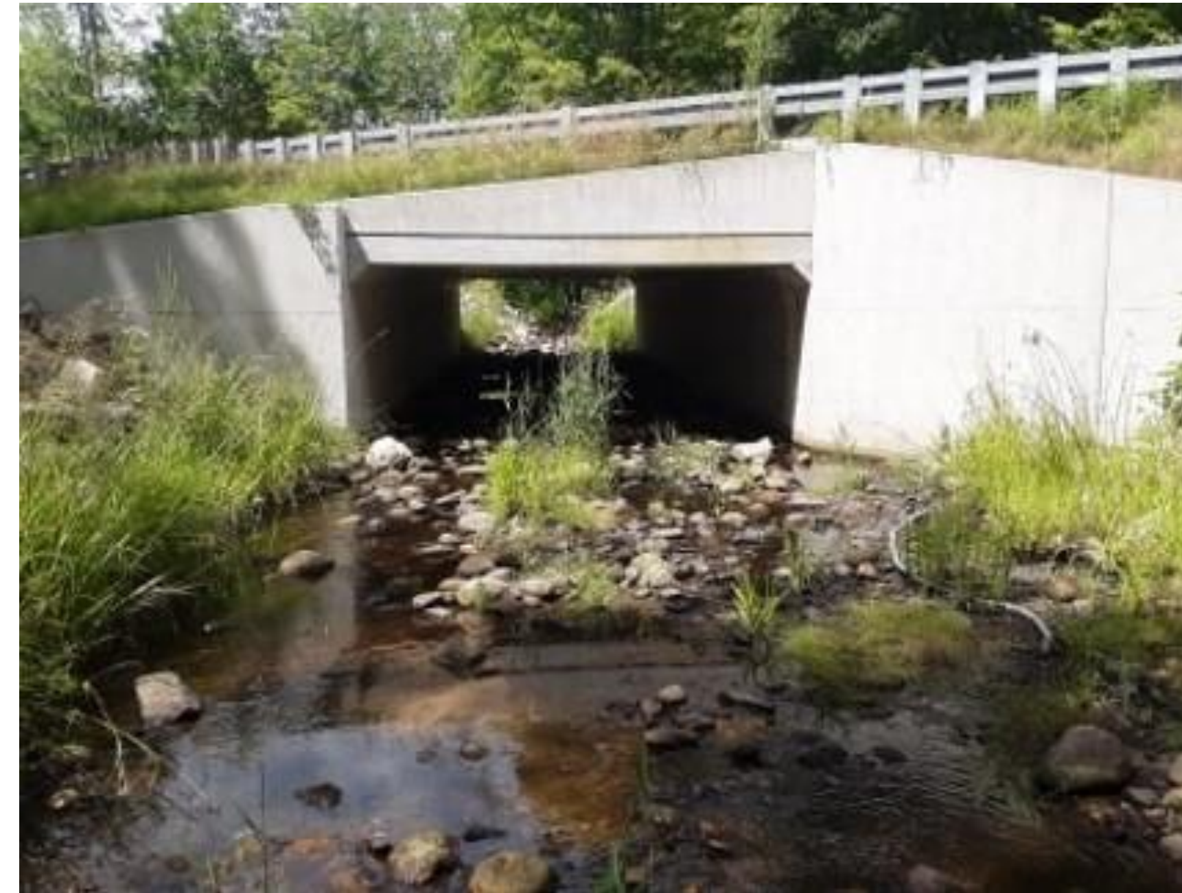
Culvert outlet performing adequately at low flow conditions, located in eastern NH
