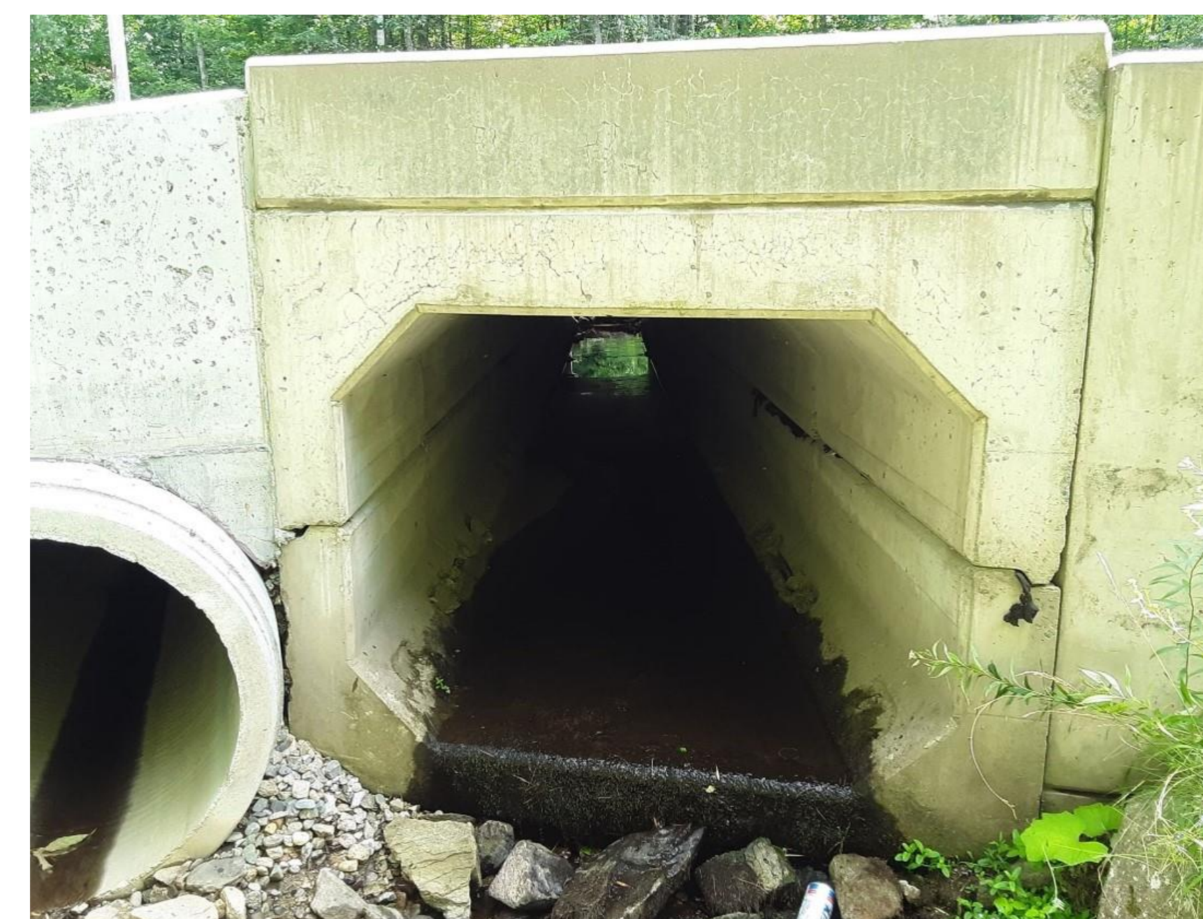
Culvert outlet exhibiting loss of bed material, located in northern NH
