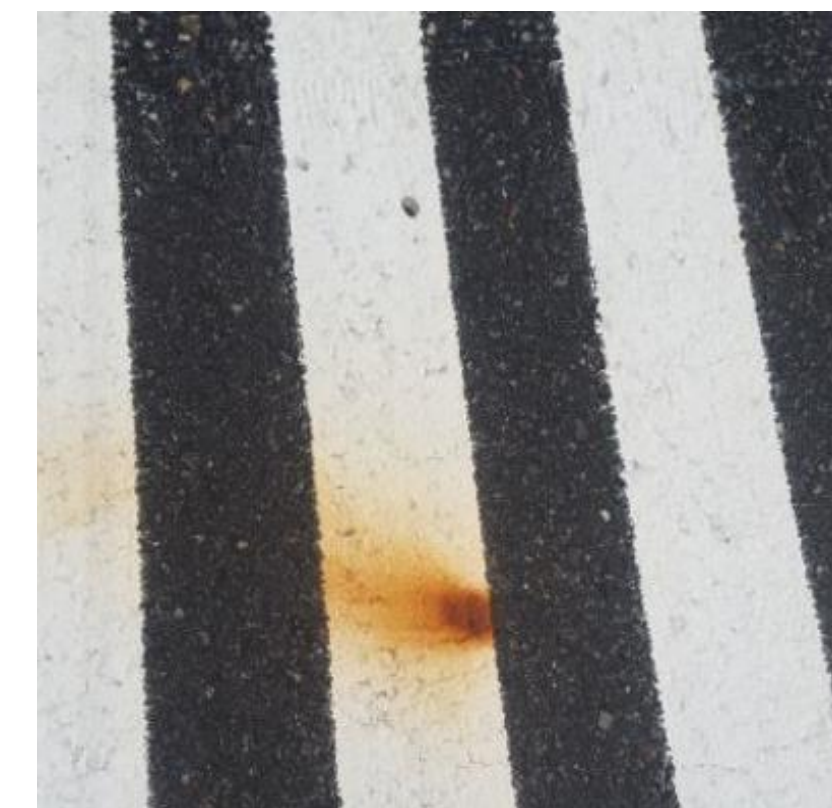
Bottom-Up Rust Stain Spot
