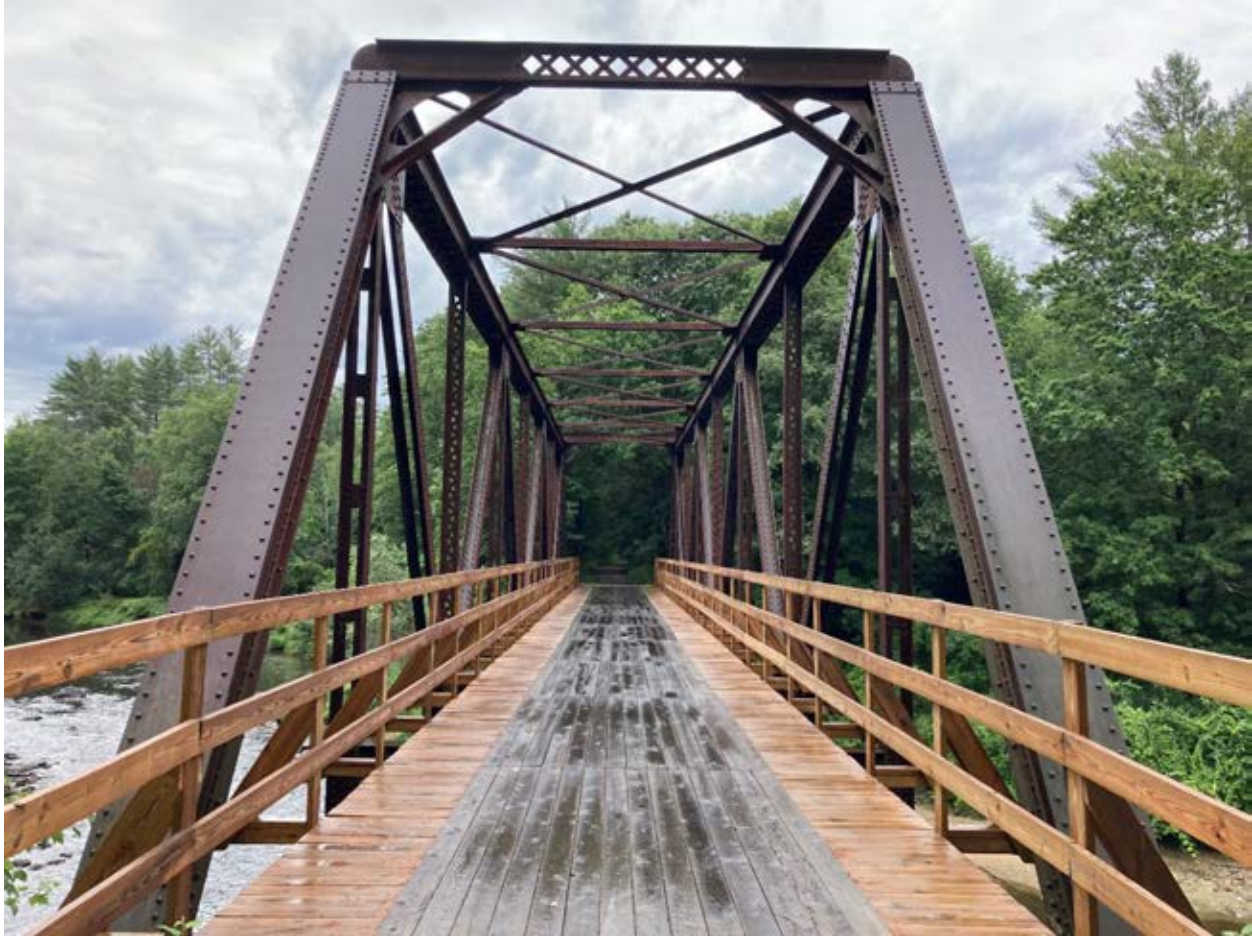
Retrofitting rail bridges for trail use is a typical rail trail improvement. (Sugar River Rail Trail, Claremont)
