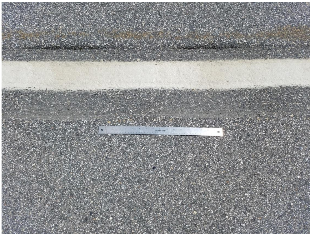
Site 1A – shoulder rumble stripe along near lane (southbound side)
