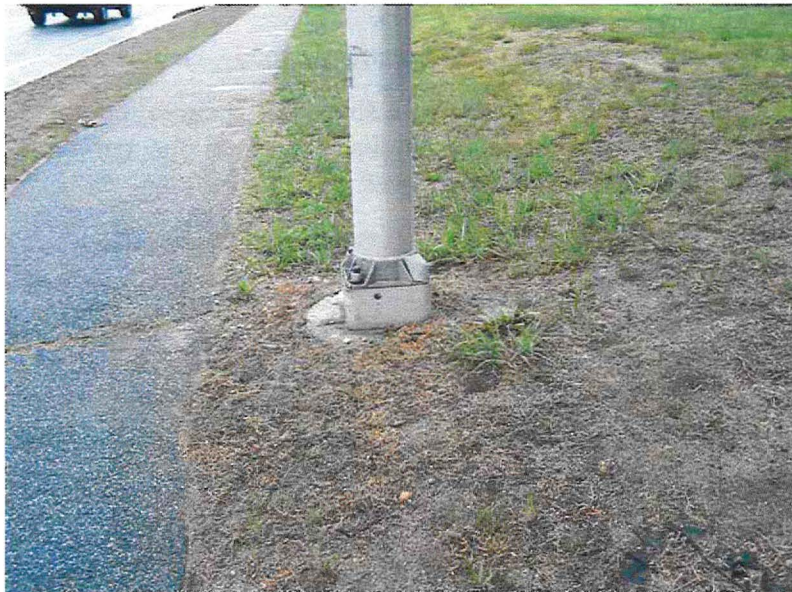
Breakaway Base- This style not commonly used in NH (Eastside Drive vic. Exit 2 –I-393 Concord)
