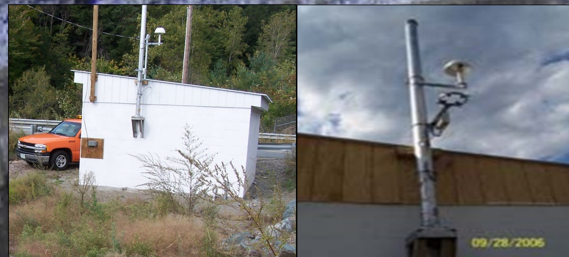
The 12'x16' pump house contains a 6,100-gal. chemical and a 300-gal. water tank, computer control equipment and an RWIS weather station to guide the system.
