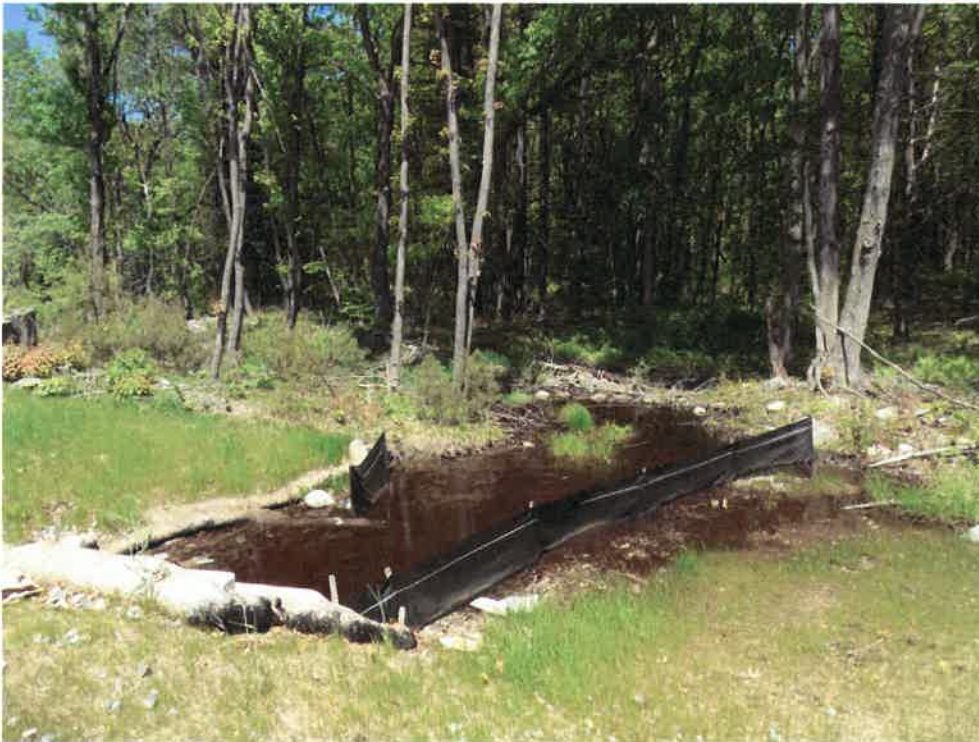
Photo 5. Facing north near southern end of Wetland 15 towards Vernal Pool 2 (5/21/2018). Erosion controls from recent construction for I-93.
