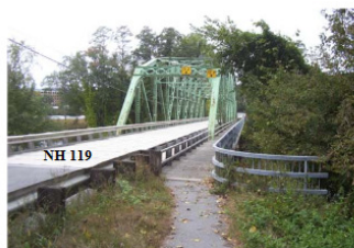
Photo PS-2 Eastern Bridge: View from New Hampshire, west towards the Mid-channel Island and Brattleboro
