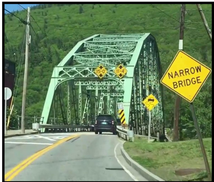
Limited Vertical Clearance and Roadway Width Limit Truck Traffic to One at a Time Crossing the Bridge
