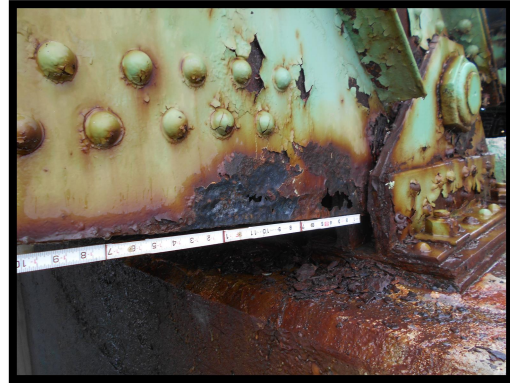
Holes through the Gusset Plate of the Charles Dana Bridge Noted in a June 2018 Detailed Inspection
