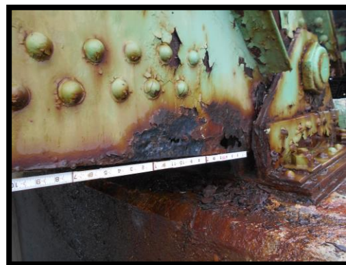
Holes through the Gusset Plate of the Charles Dana Bridge Noted in a June 2018 Detailed Inspection
