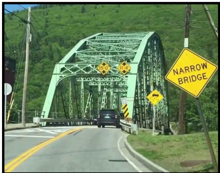
Limited Vertical Clearance and Roadway Width Limit Truck Traffic to One at a Time Crossing the Bridge
