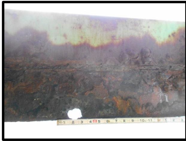
The superstructure condition rating of the bridges was recently reduced to a 4 (Poor) and Remedial Repairs may be required. (Photo – Hole in Lower Chord June 2018 in Charles Dana Bridge)
