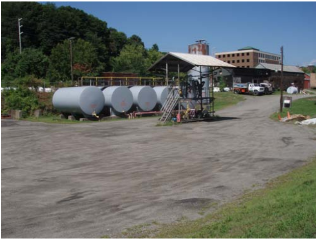
Photo 13 – Bulk Fuel Tanks
