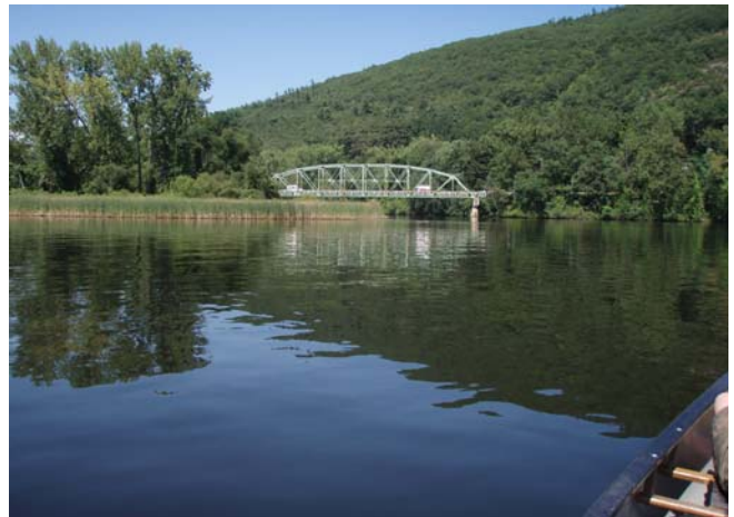
Photo 4 – Route 119 Easterly Bridge View of the Route 119 Easterly Bridge from the Connecticut River northeast towards New Hampshire.
