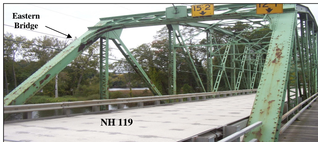
Photo B-7 Eastern Bridge: View from New Hampshire, west, towards Vermont. (note: Bridge clearance is currently 14’-10” at the center and 11’-10” at the exterior)
