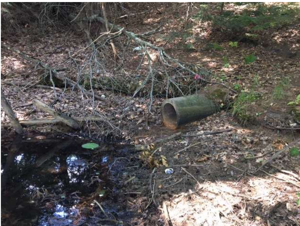
Photo 6: Impact Locations F, G, and H (WB) Drainage Outlet at Harris Pond
