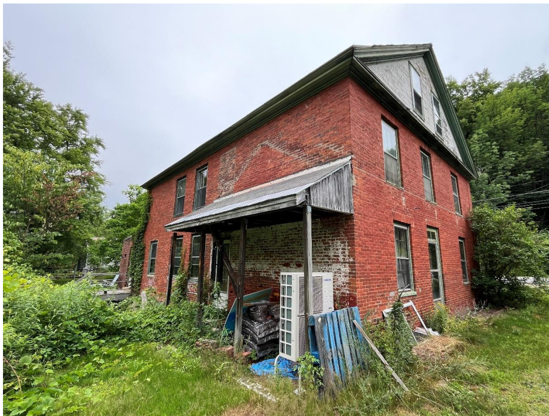
Photo # 9: Rear elevation of Rixford House. Note ghosting of ell gable and infilled window. Looking N.
