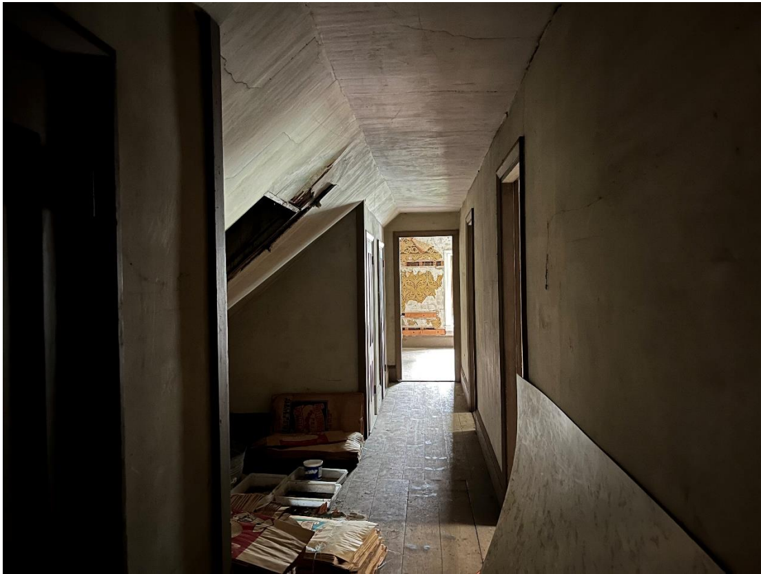
Photo # 22: Third floor hallway of boarding house, looking NW toward gable end room. Closets on left.
