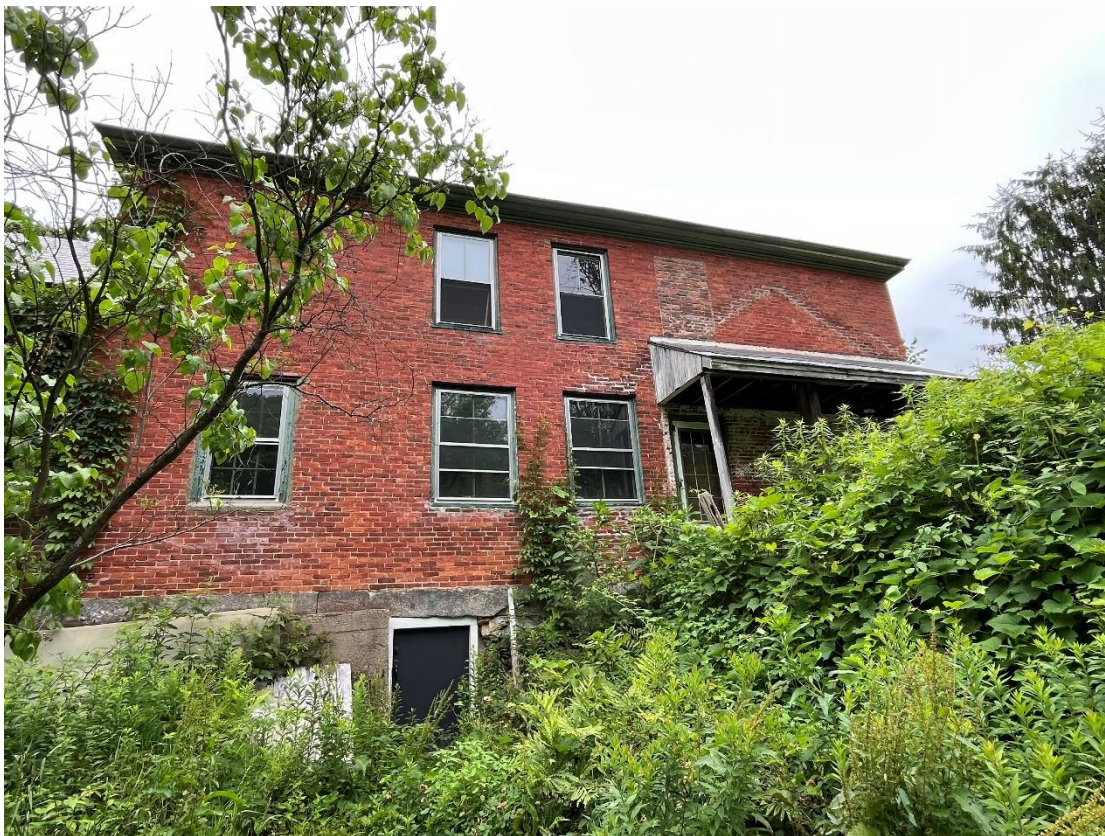
Photo # 10: Rear elevation of Rixford House, looking NE. Note widened windows on the first floor.
