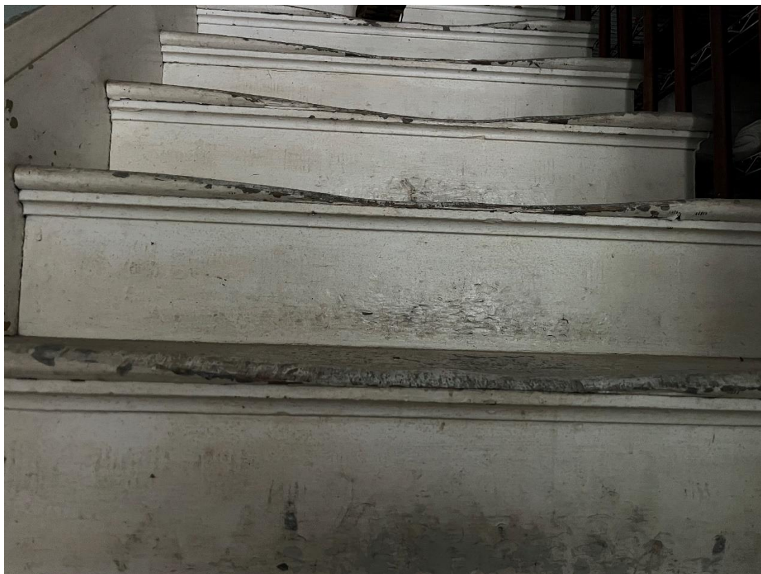
Photo # 17: Worn stair treads in boarding house wing. Looking W.
