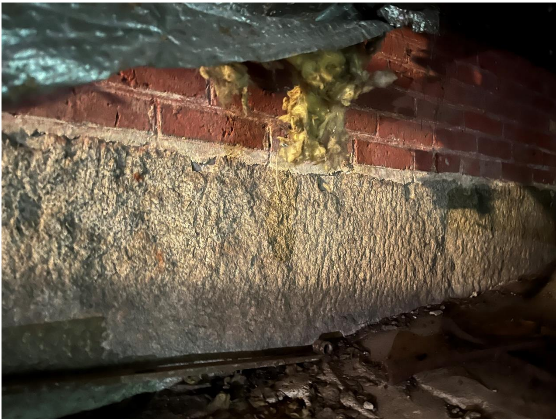
Photo # 25: c.1825 split marks on the Rixford House granite capstones.
