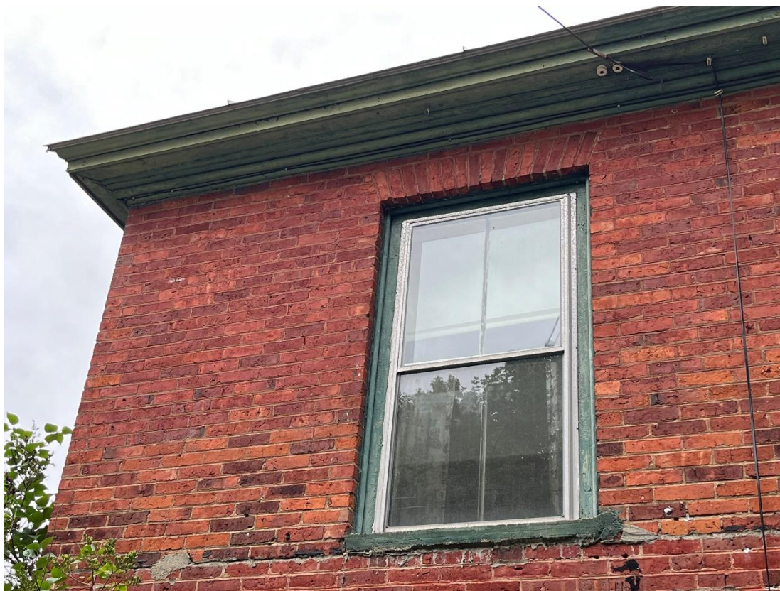
Photo # 12: Detail of bed molding, window casing, and brickwork of Rixford House, eastern corner. Note the concrete window sills. Looking SW.
