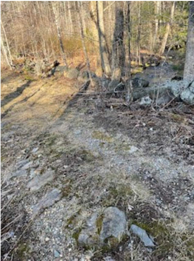
Photo #6 Stones in the roadbed taken facing northeast standing on the roadbed. 5/6/24
