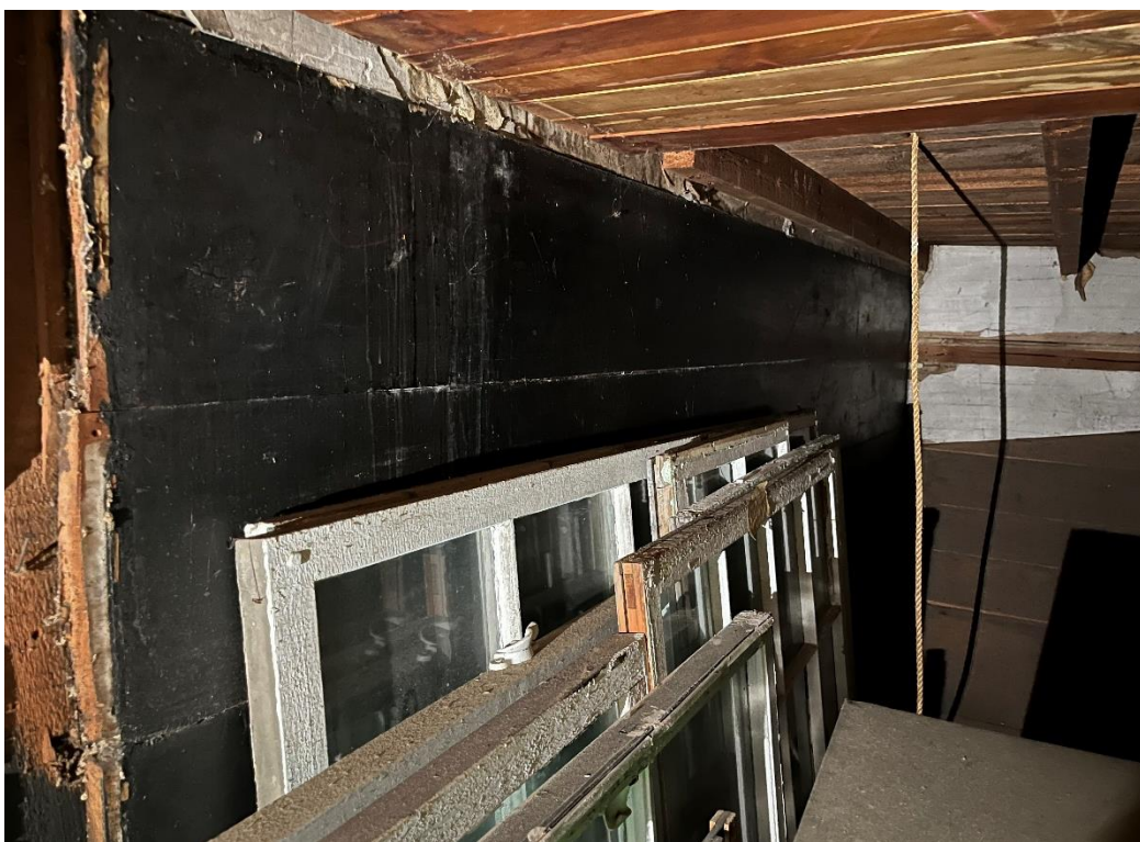
Photo # 11 Description (with direction): Interior, second floor, looking NW at original blackboard, now hidden in storage closet.
