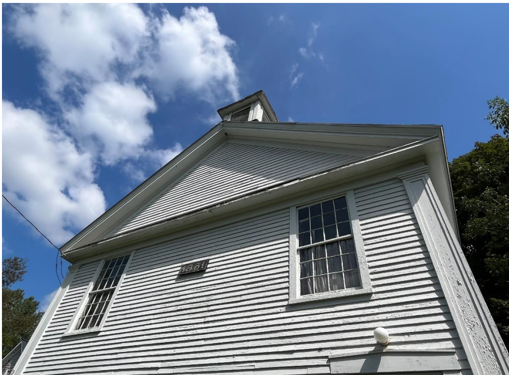
Photo # 7 Description (with direction): Detail of façade's gable end and corner pilasters. Looking NE.
