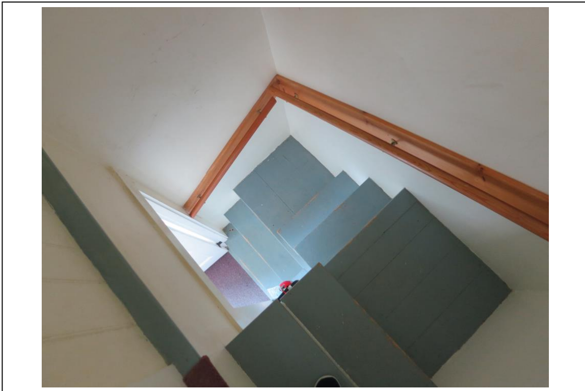
Photo #11 Description: Looking down stairs from gallery at west corner of building
